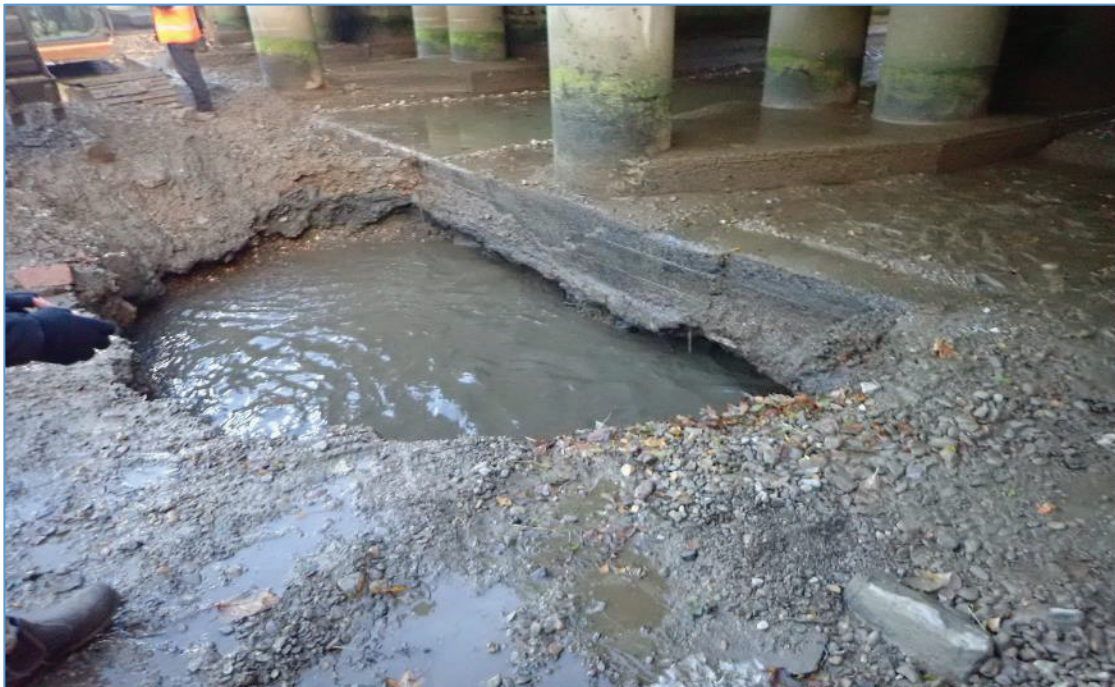
Plate 28: TP-05, view from the west, showing the extent of the area opened upstream of the bridge, exposing the concrete plinth added as part of the bridge-widening works in the 1970s.
