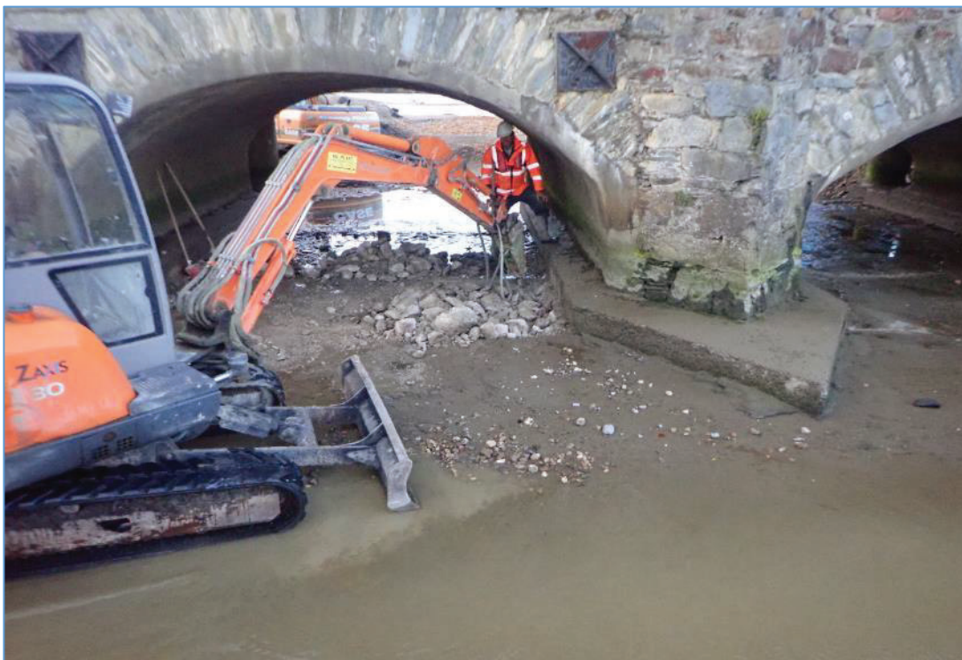
Plate 9: Record shot of the rock-breaking employed to break through the apron at the trail pit locations.
