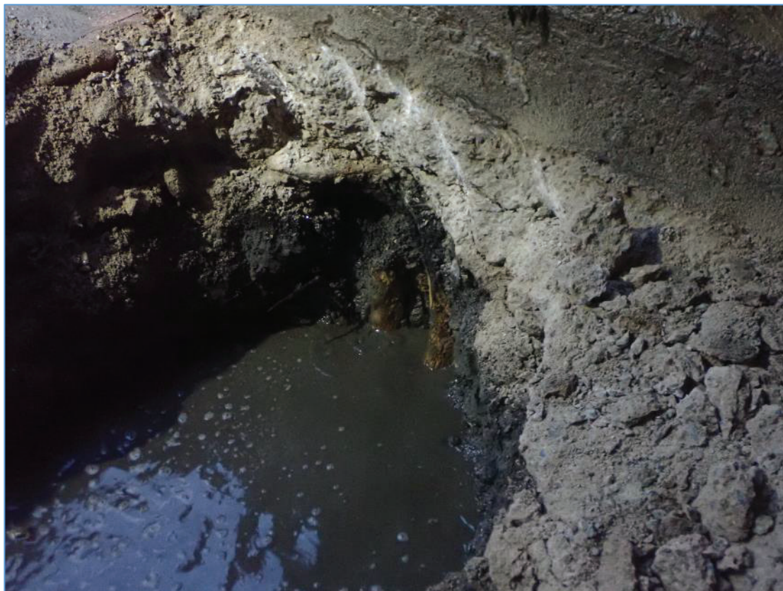
Plate 22: TP-03 at Pier 2. Removal of the covering concrete reveals river clay and starling piles.
