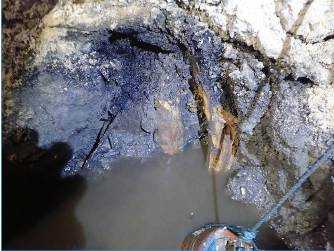
Plate 23: TP-03 at Pier 2, close-up view of the starling piles to their excavated depth.
