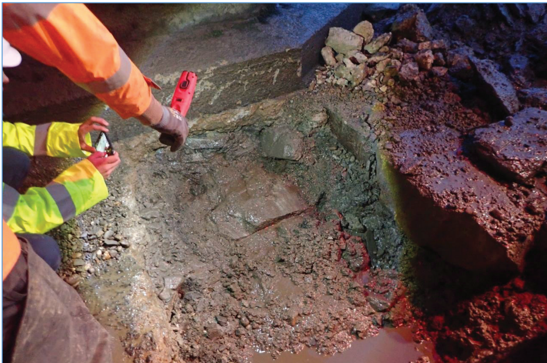
Plate 23: TP-02, view showing the stone of the bridge apron exposed below the more recent concrete layer above.
