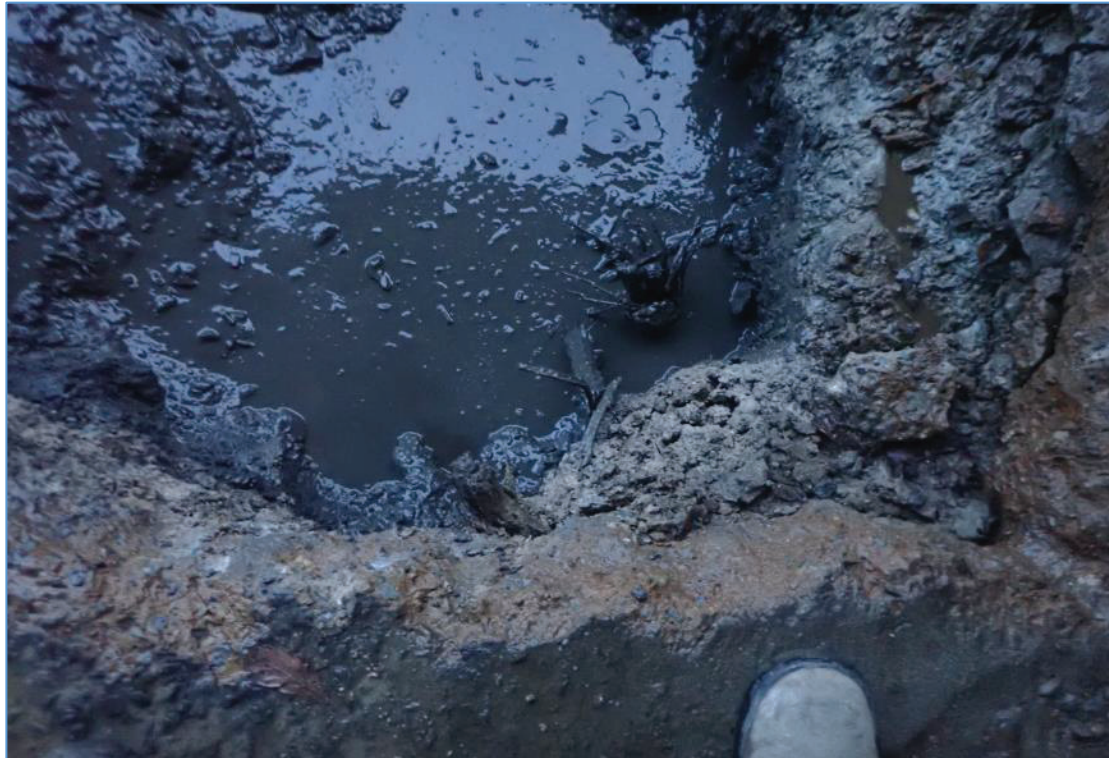
Plate 37: TP-02 at Pier 1. Excavation of the covering concrete layer revealed the tops of large stone and timber fragments.
