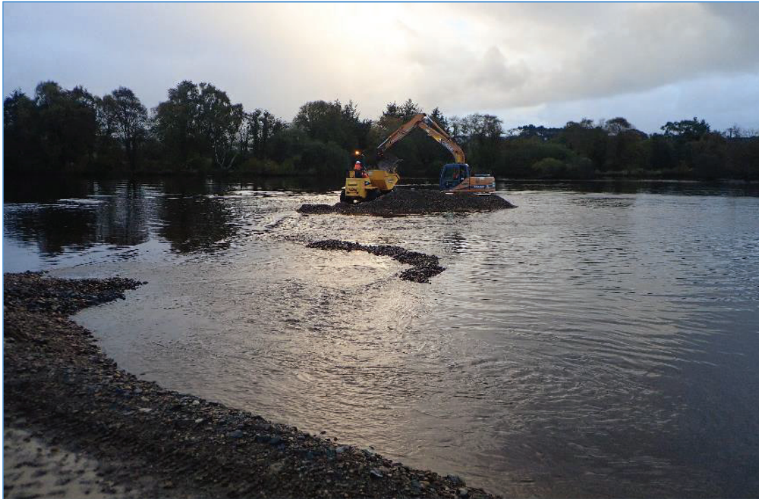
Plate 4: Excavation of the shingle bar that forms naturally upstream of the bridge, which was the source of the shingle used to create the access road and river bunds.
