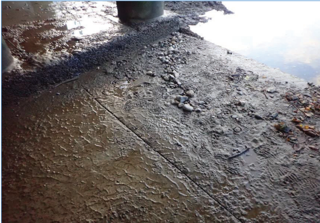
Plate 8: Record shot of cut through the apron between the piers in preparation for excavation of the trial pits.
