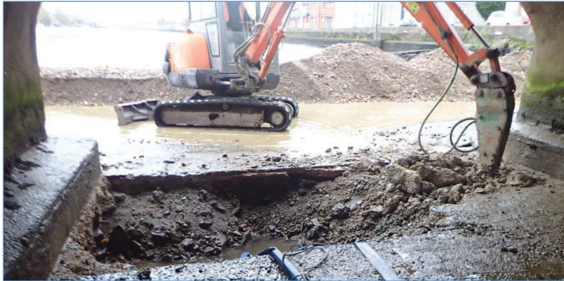
Plate 24: TP-03 as it was being excavated across the space between the bridge piers, reveals the shallow nature of the concrete added above the stone apron.
