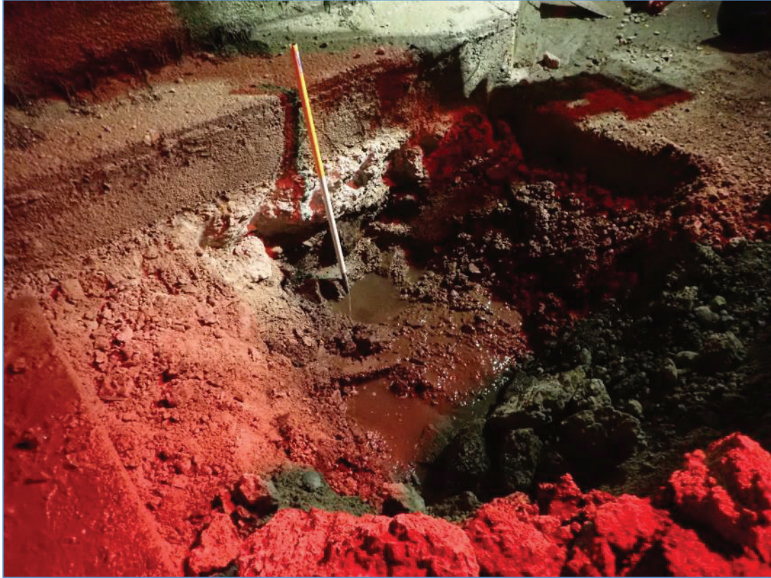
Plate 19: TP-03. Excavation of the concrete above the bridge apron at Pier 3 reveals the apron's stone.
