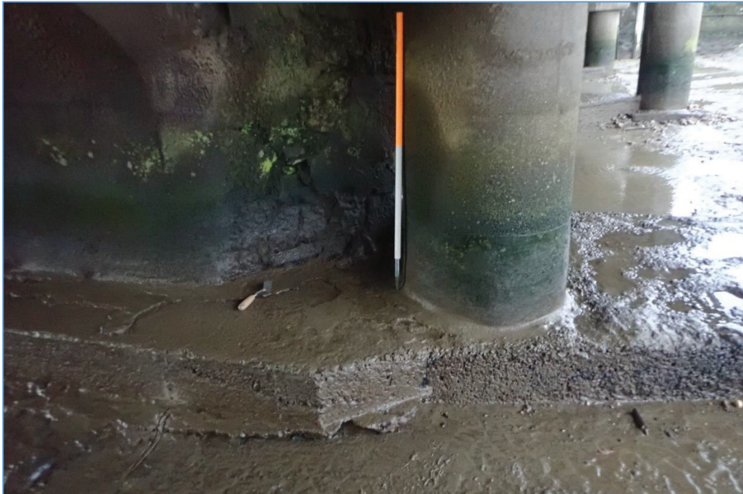
Plate 29: Pier 3, east-facing side, showing the join where the bridge-widening works of the 1970s is added to the concrete surround to the earlier stone pier. This presents a stratigraphic sequence of the bridge works in the modern period.
