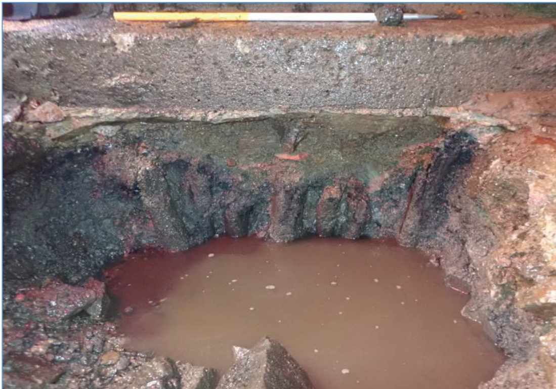
Plate 24: TP-04 at Pier 4. Excavation reveals a line of starling piles under the stone apron.
