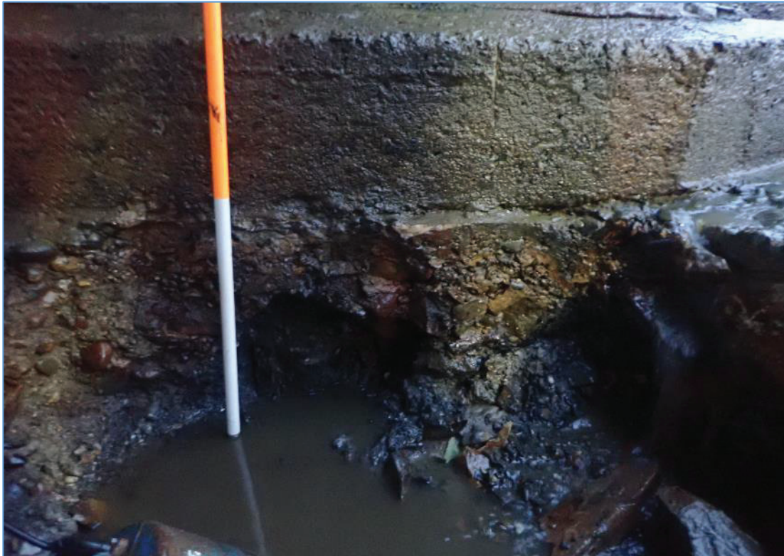
Plate 27: TP-04 at Pier 4. Excavation revealed starting piles under the stone apron that in turn lies under the more recent concrete that forms the current bed level.
