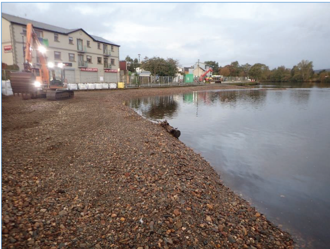
Plate 5: View looking upstream of the access route created along the west bank from river shingle.
