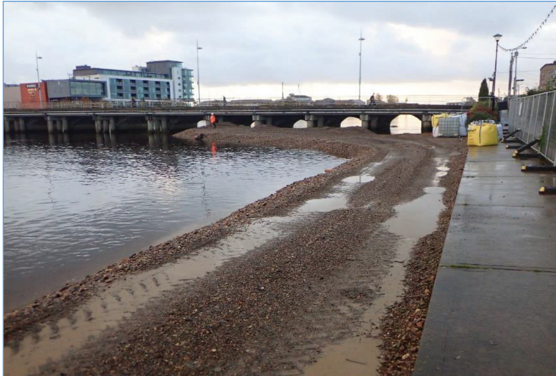
Plate 6: View looking downstream showing the access route and upstream bund created from river single.
