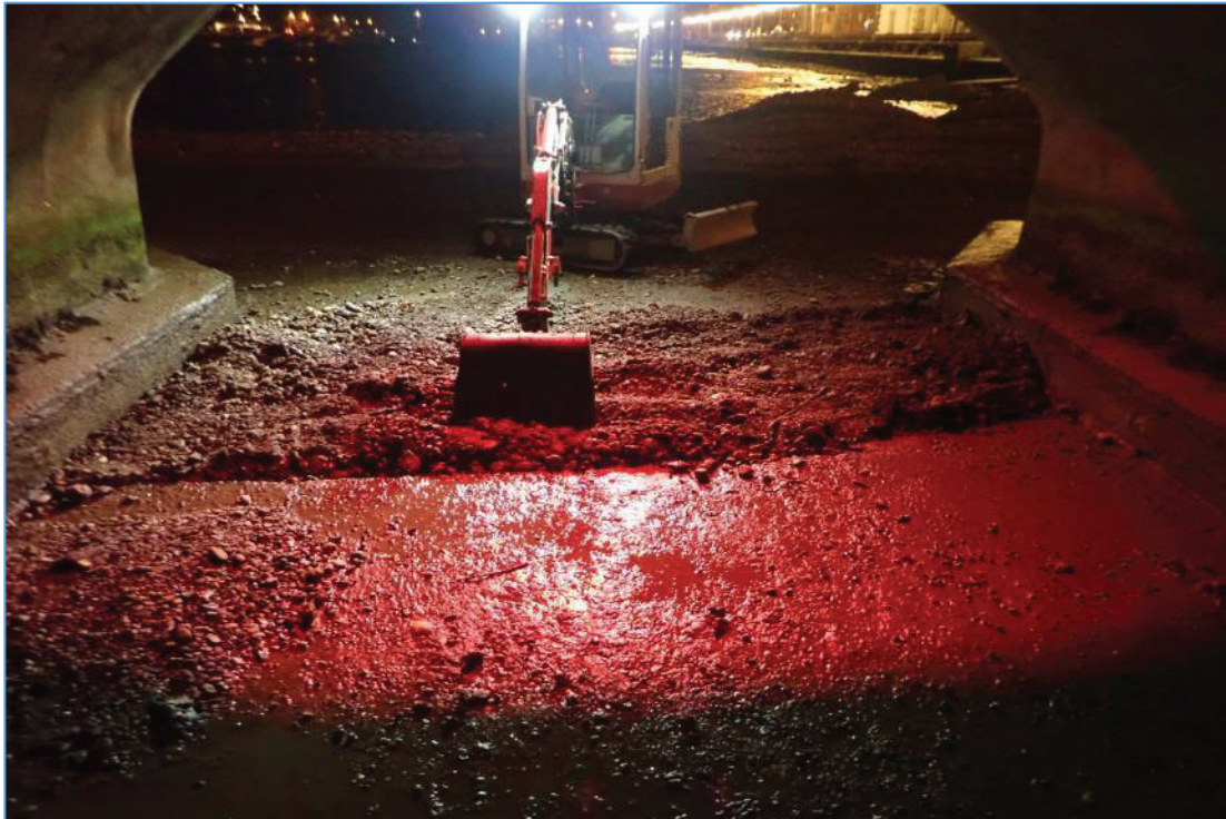
Plate 10: Record shot showing the back-filling of the trial pits. This would be replaced later with a concrete solution on completion of the SI work.
